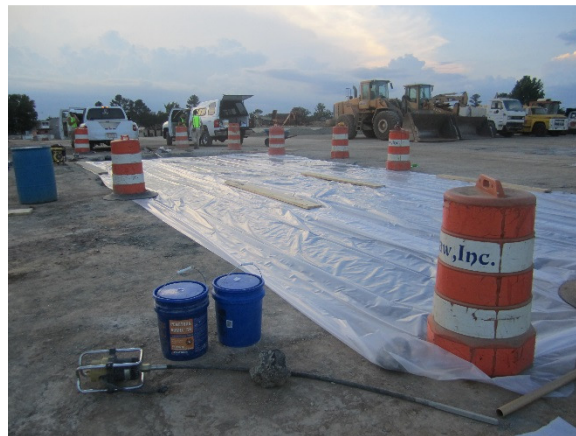
Figure 6. Curing of the finished RBMAC test pavement (foreground) and conventional PCC control pavement (background)
